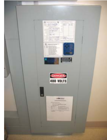
Figure 24: 480V AC Electrical Panel (interior)
