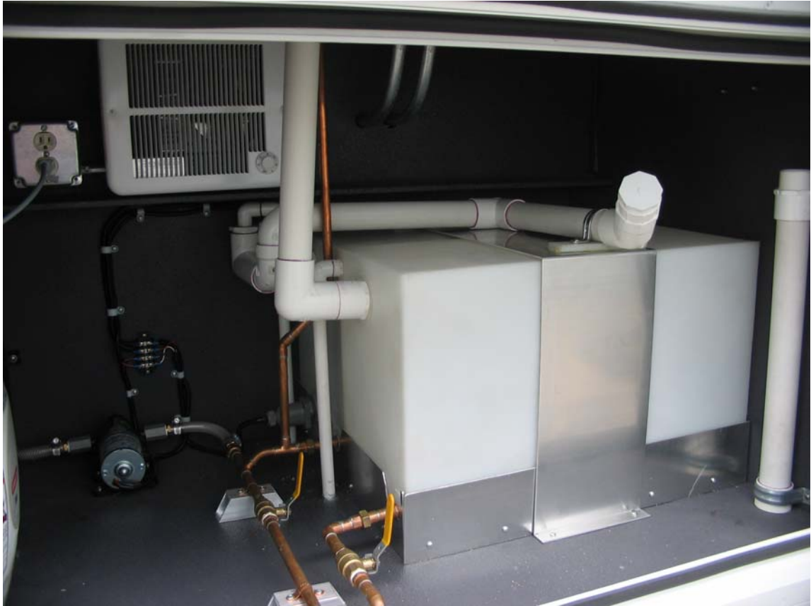
Figure 32: Fresh Water and Wastewater Compartment
