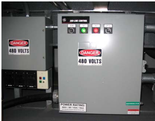
480V AC Switching Panel
