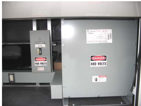
480V AC – 208/120V AC Transformer and Control Breaker
