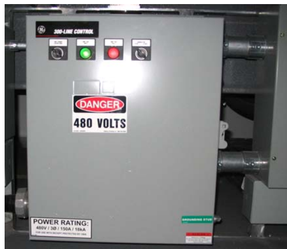
Figure 21: AC Electrical Power Source Control Panel
