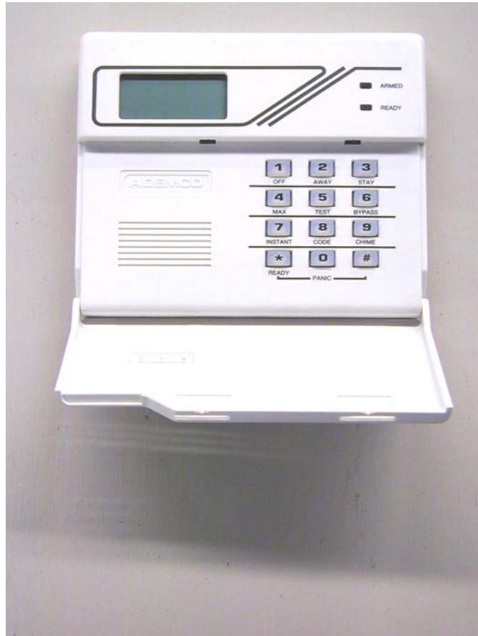
Figure 40: Intrusion Alarm Keypad
