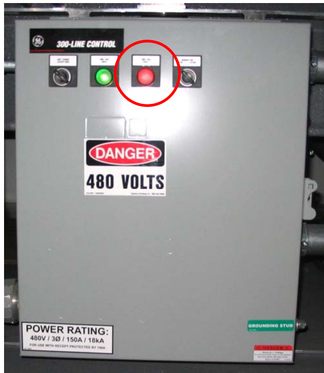
Figure 48: 480V AC Fault Indicator Light
