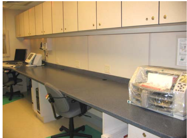
Figure 4: Control Room Overall
