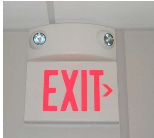
Figure 44: Emergency Dual Beam Lighting
