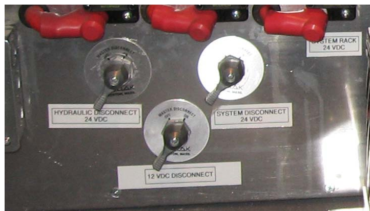
Figure 13: Power Disconnect Switches DC
