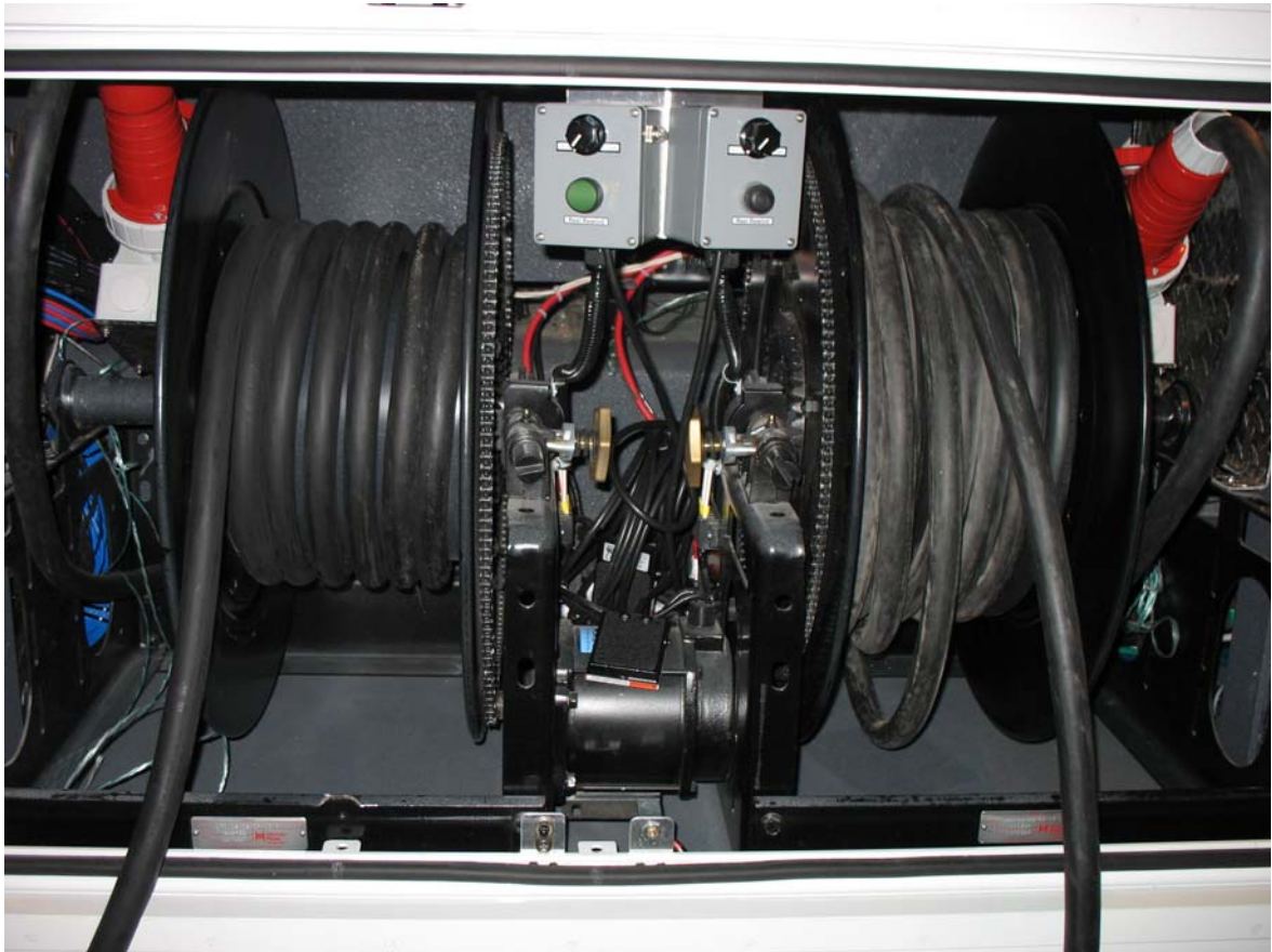
Figure 10: Shore Power Cable Reels & Controls
