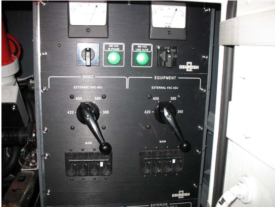
Figure 11: Power Input Panel
