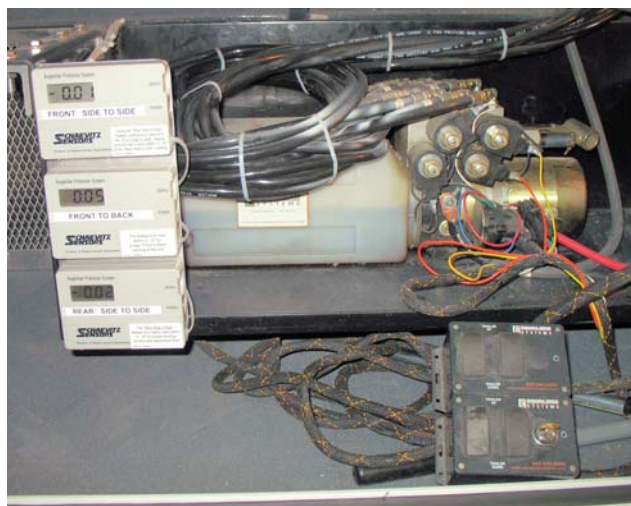
Figure 7: Landing Legs Hydraulic Power Unit
