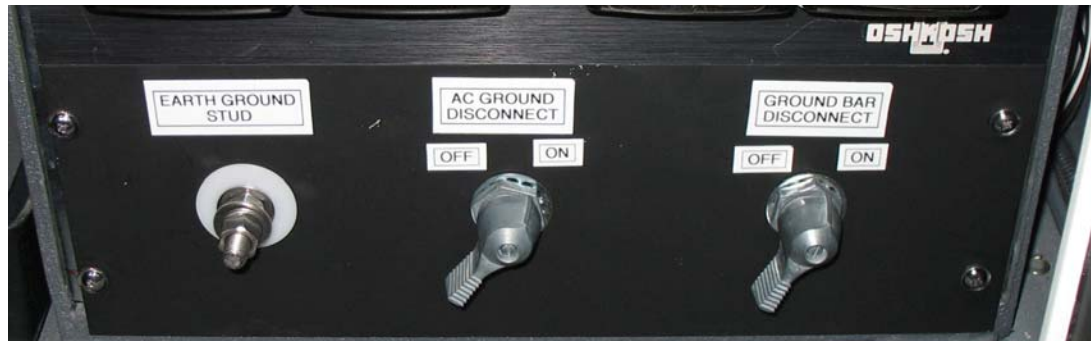
Figure 6: Ground Stud and Disconnect Switches
