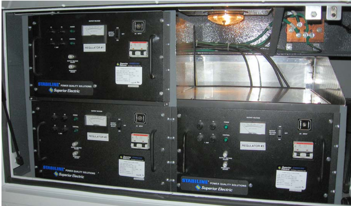
Figure 12: Power Conditioner Regulators
