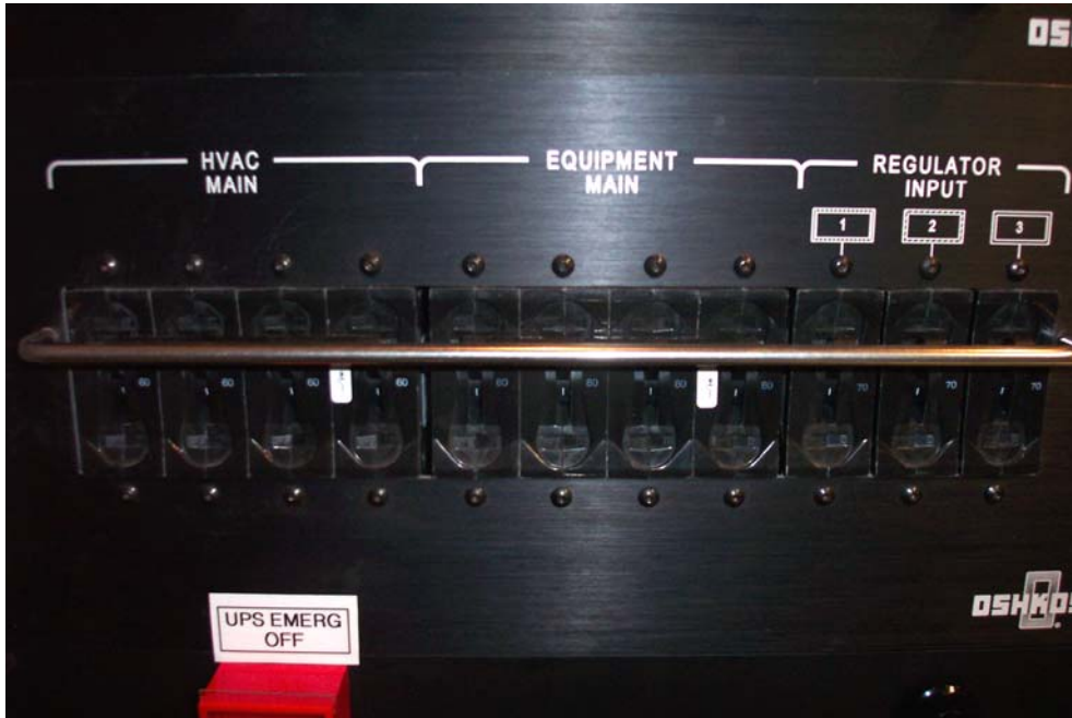
Figure 14: Power Distribution Main Panel
