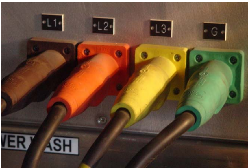
Trailer Underbody Power Connections
