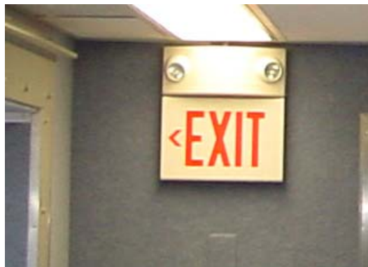
Command Room #3 Emergency light
