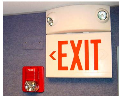
Communications Room #1 Emergency light
