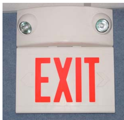
Command Room #2 Emergency light
