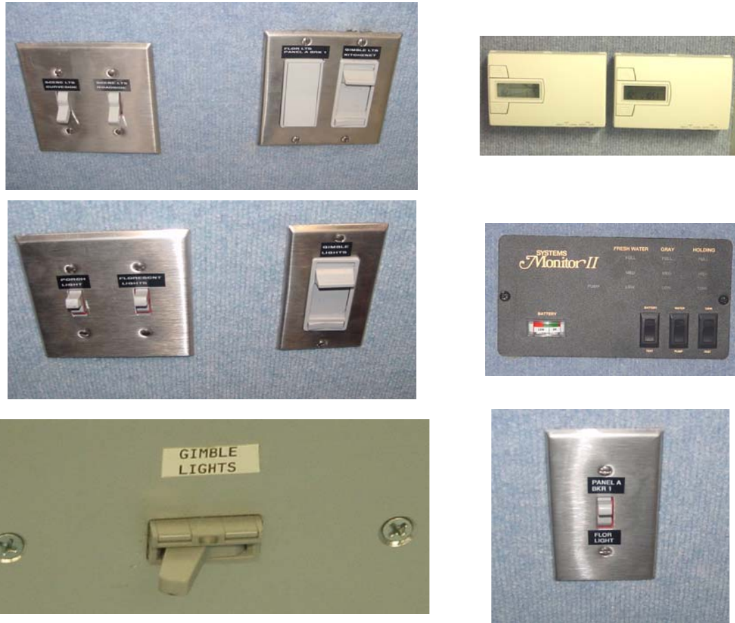
Figure 11: Mobile Unit Controls
