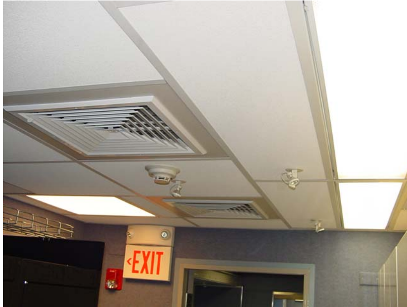
Figure 40: Communications Room #1 Overall Lighting
