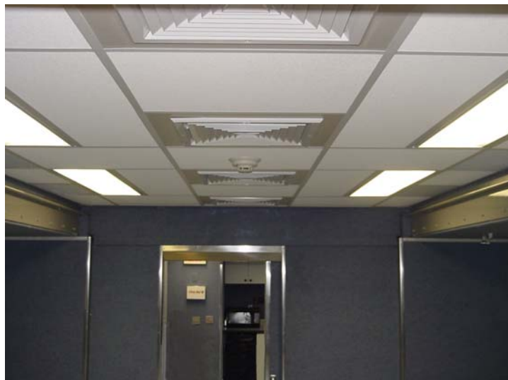
Figure 39: Command Room #2 Overall Lighting
