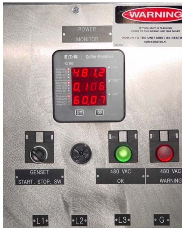
Figure 27: 480V AC Phase Power Monitors
