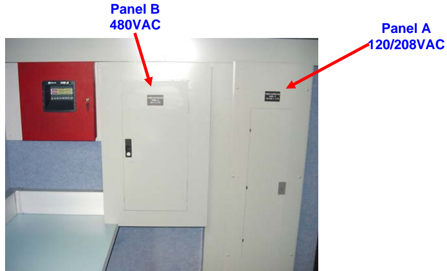
Figure 25: 480V and 120/208V AC Electrical Panels
