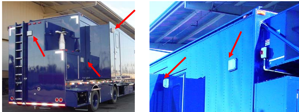
Figure 36: Entry Door Lighting
