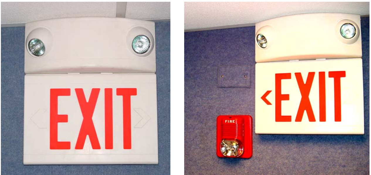
Figure 2: Emergency Lighting (Typical)
