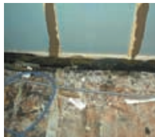
Interior Water Damage
