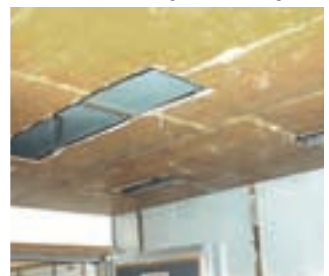
Water Damage to Ceiling
