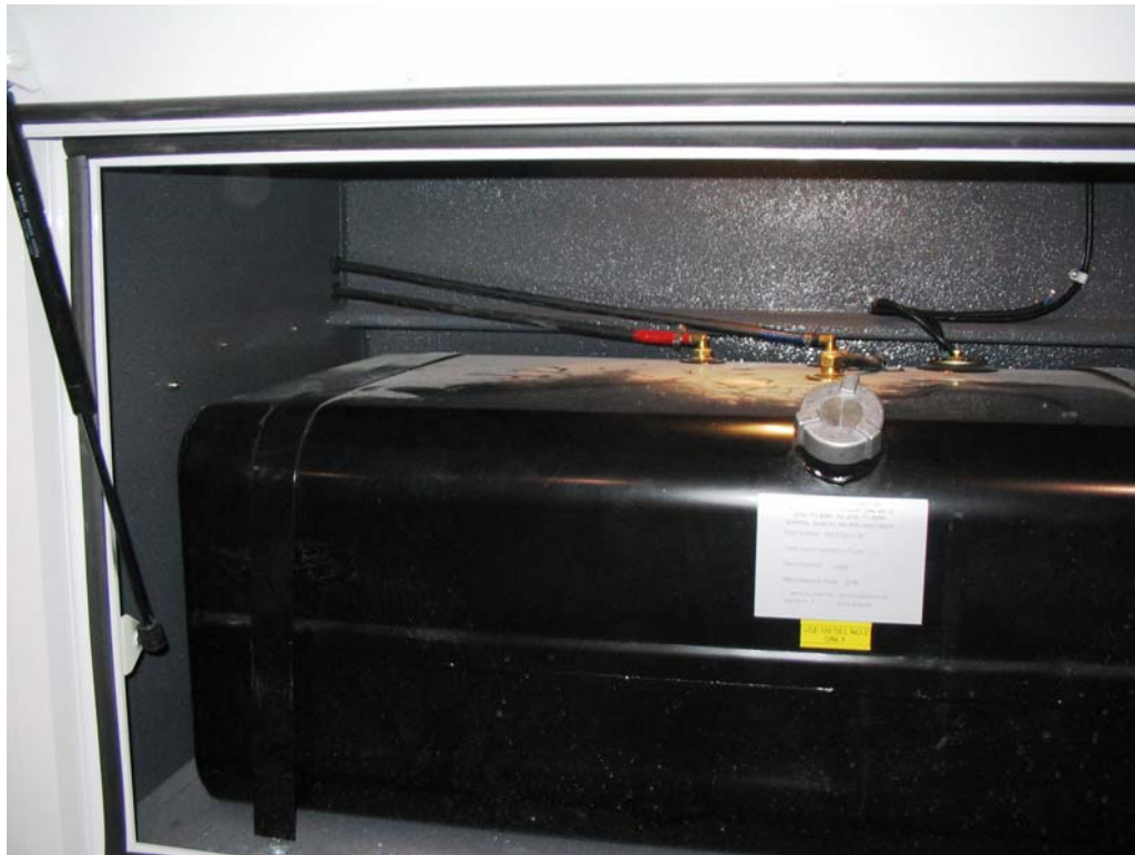
Figure 1. Lower Tank Compartment Prior to Installation
